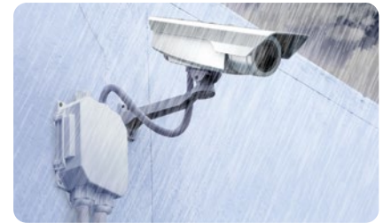
Installation with free cables.
