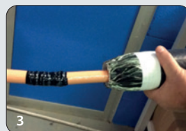
3 Position at the centre of the connection and collapsed on the cable removing the inner support.
