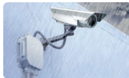
Installation with free cables.
